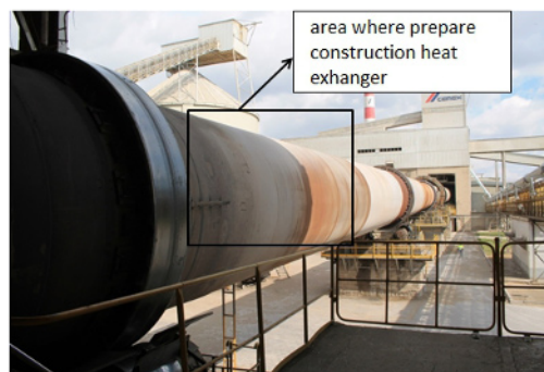
Figure 4. Rotary boiler number 4
