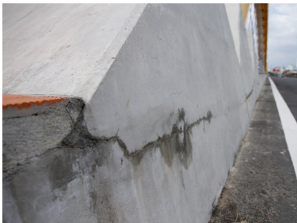
Figure 16. Cracks appeared in the abutment after construction.
