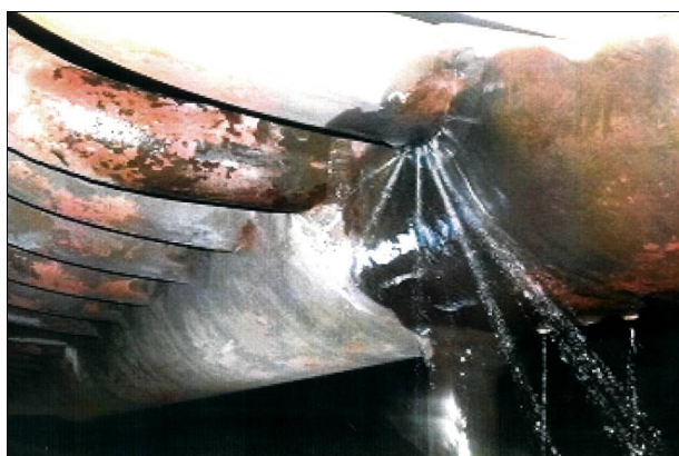
Fig. 10. Indirect (lower) HP superheater II header – fillet weld damage.
