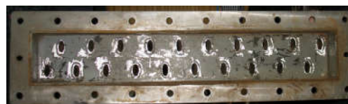
Fig. 12. A view of sieve plate and its connection with heat exchanger header
