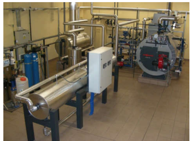
Fig. 6. View of the experimental installation for testing the computer system for on-line monitoring thick-wall pressure components
