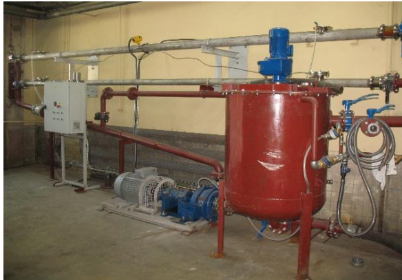
Fig. 4. General view of the salt debris leaching system.
