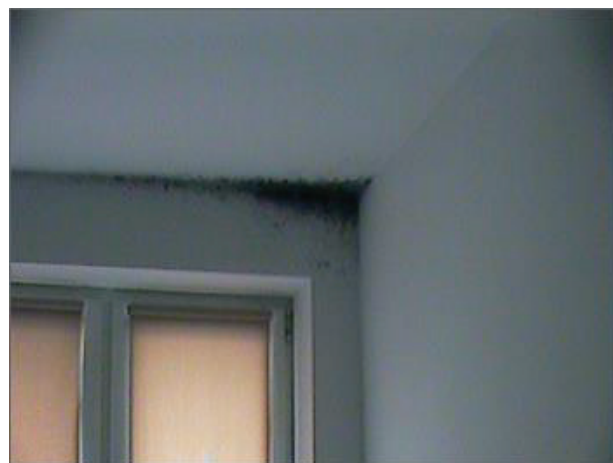
Fig. 7. Detected troubles in the tested residential apartment buildings: mold in the room corner, on the internal surface of the external wall, caused by limited infiltration of external air, poor natural ventilation, thermal bridges and significant moisture gains from people.
