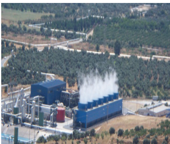
Fig. 8. An image of the cooling system of GEPP's.
