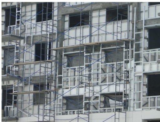
Fig. 3. The protecting constructions of the high-rise building with filling a foamconcrete into the fixed formwork.
