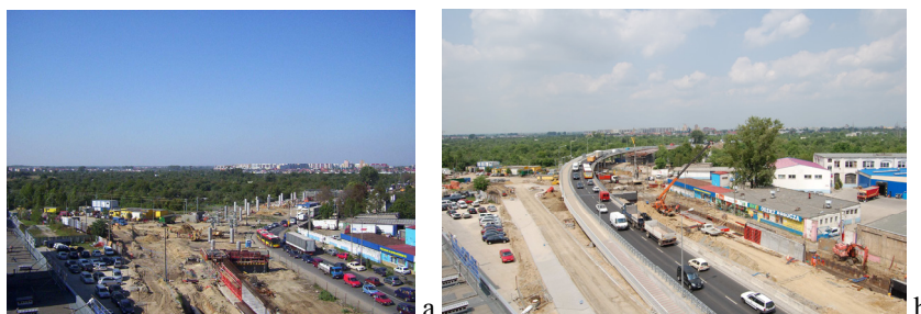
Fig. 8. The process of formation of a flyover over Klecińska Street as part of the "Downtown Ring Road" section (a - September 2006, b - May 2007), photo: author.
