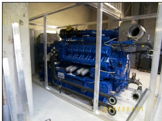
Fig. 3. Trigenation power plant at Campus Luigi Einaudi.
