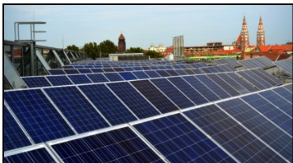
Fig. 4. Solar panels at the roof of SZTE TIK
