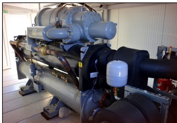
Fig. 3. Heat pump for usage of wastewater heat
