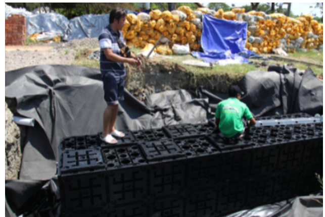
Fig. 4. Urban farming ITS products and underground tanks to harvest rainwater
