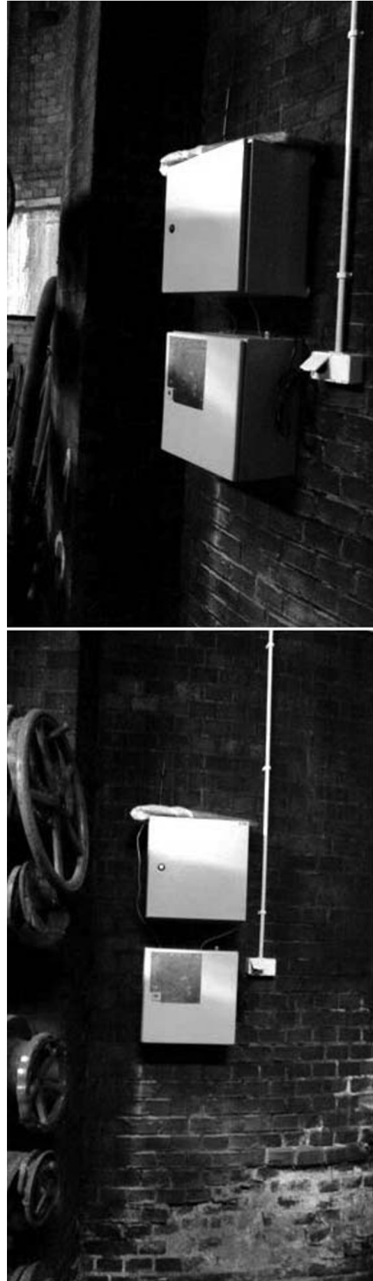
Fig. 5. The place of sensor installation.
