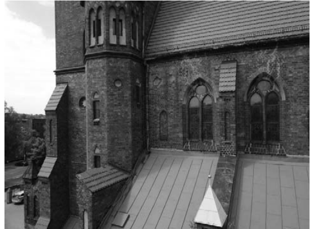
Photo 7. The Eastern wall of the church nearby tower (fissures and rosette deformation).
