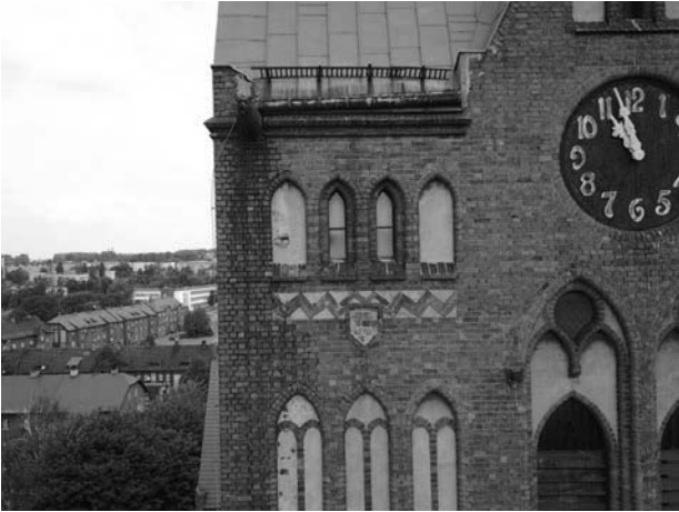
Photo 4. View of the church tower, close-up on the upper part of the tower for inspection of damages in the wall.
