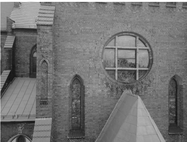
Photo 6. View of the western wall of the church nearby transept (vertical fissures).
