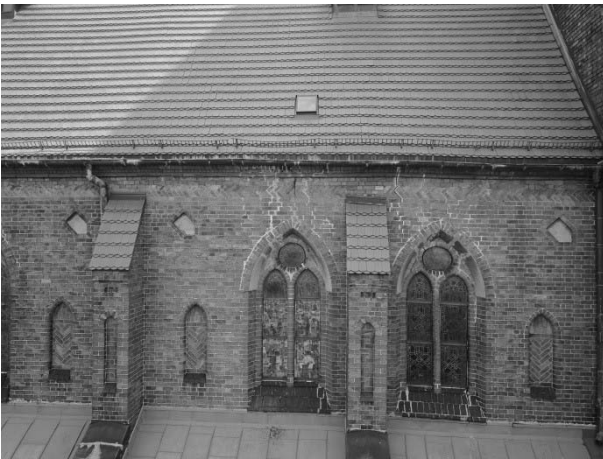
Photo 5. View of the western wall of the church nearby tower (cemetery side), visible fissures and rosette deformation.
