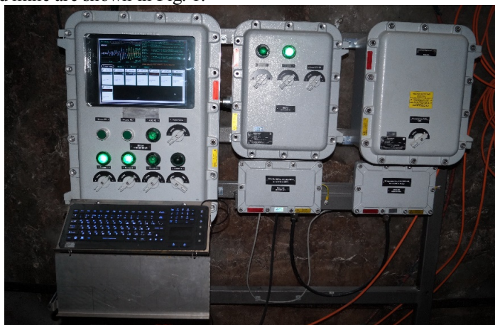
Fig. 1 - Explosion-proof switching and distribution unit "Prognoz-ADS" automated system (PB Ex d I Mb)
