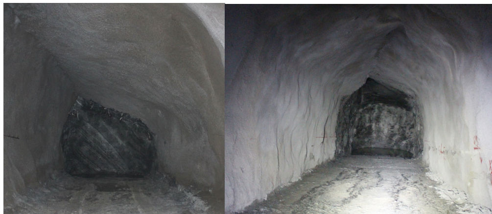
Fig. 4 Brittle outline fracturing at the mines of Kirovsk branch of JSC "Apatit".
