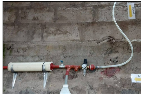
Figure 9. Biogas outlet, filter and valve unit.
