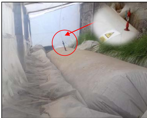
Fig. 8. Biogas output piping from the Biodigester.
