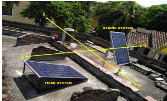
Fig. 1. Location and installation of fixed and hybrid system.
