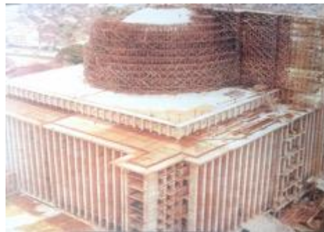
Fig. 3. The Construction Process of Istiqlal Mosque Dome. Source A. Armand et. Al., 2014
