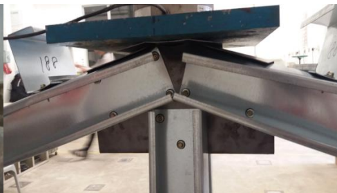
Fig. 10(b). Distortional buckling of top chord for conventional truss specimen.
