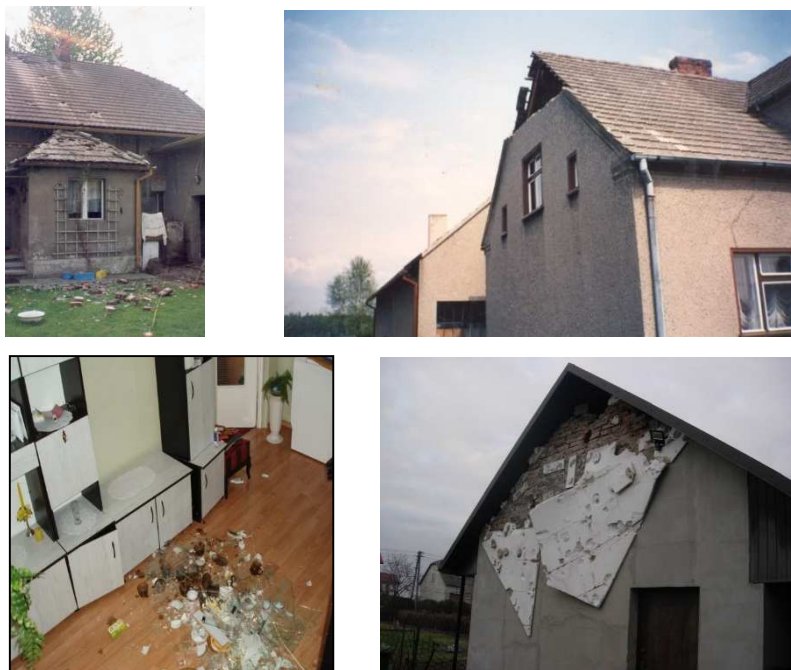
Photo 1. Damage in buildings after a tremor of seismic energy E = 1 \cdot 10^9 J, M_L = 3.8 ).
