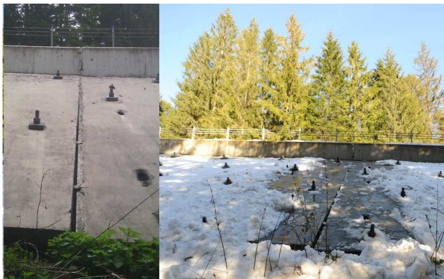
Fig. 3. Retaining structure with the damaged slab section (photo by authors).
