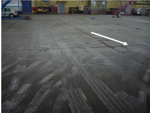
Fig. 1. The inside of the hangar. Damages to the floor are visible.
