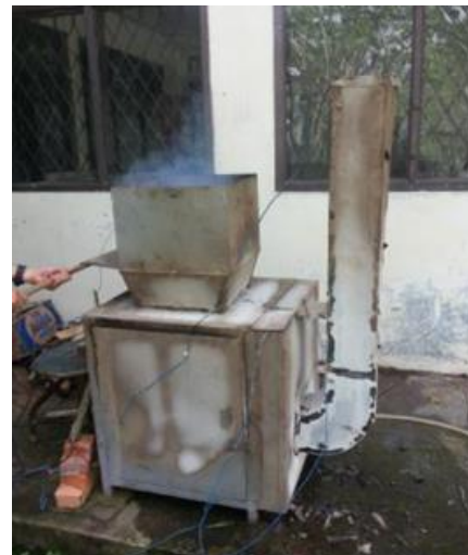
Fig. 3. Continuous type incineration
