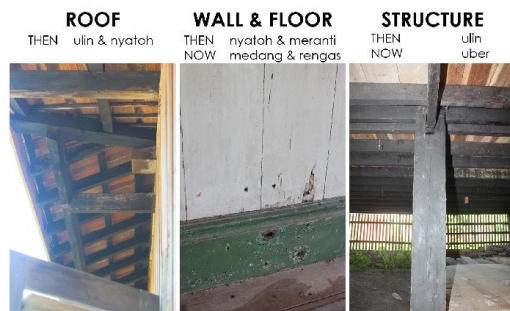
Fig. 3. Various types of woods in constructing traditional stage-houses in Bangka, which influenced by Palembang’s pyramid roof (source: Findanavy and Syahid, 2018).
