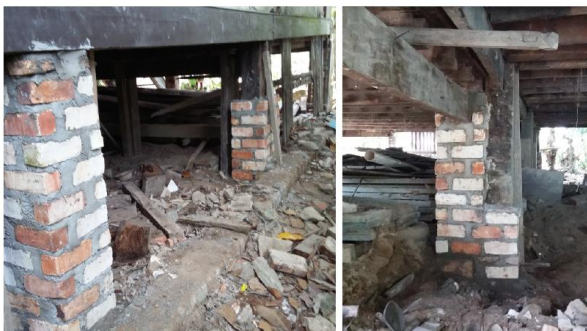
Fig. 4. Reinforcing the structure of a traditional stage-house by replacing or integrating the decayed wood with concrete and bricks (source: Yana, unknown year).
