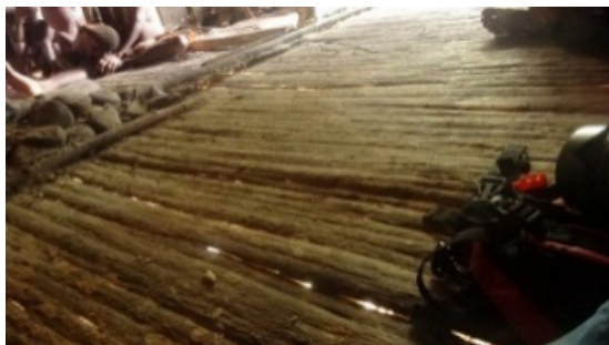
Fig. 9. Nibung as floor-covering.
