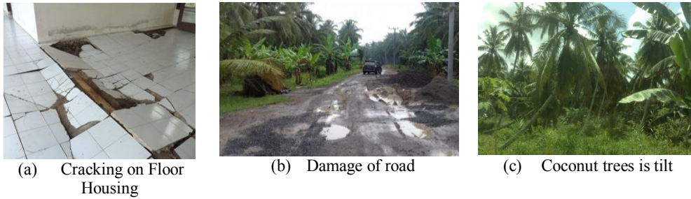
Fig. 4. Direct Impact of Land Subsidence.
