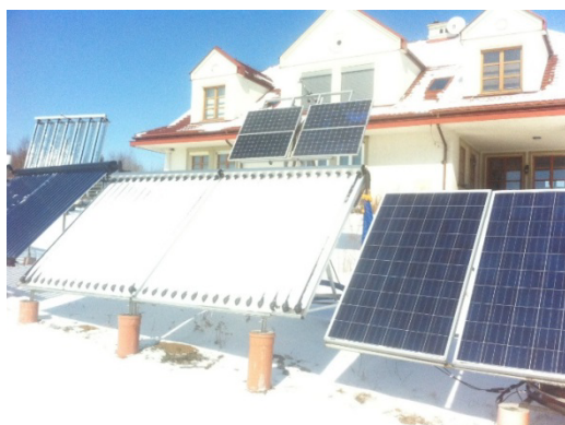
Fig 4. The ST and PV arrays in front the house in winter.
