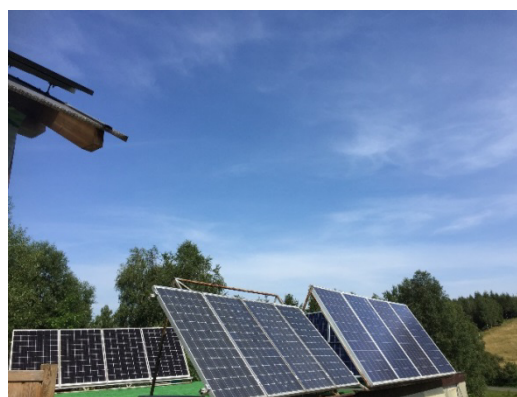
Fig 5. The PV arrays standing on the ground and the top of garage.
