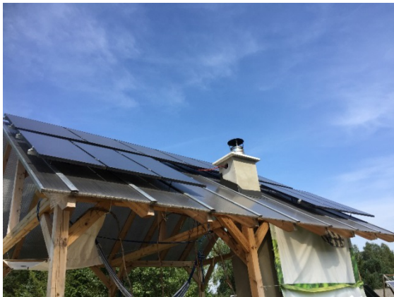
Fig. 2. An extra PV panels deployed in the second scenario at the roof top of a garage.
