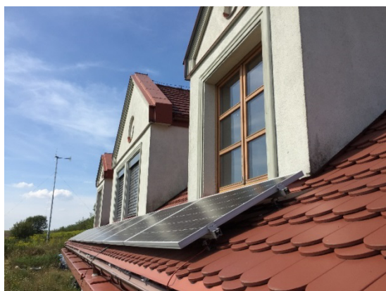
Fig 3. The house with PV mounted at the roof at the first stage of experiment.
