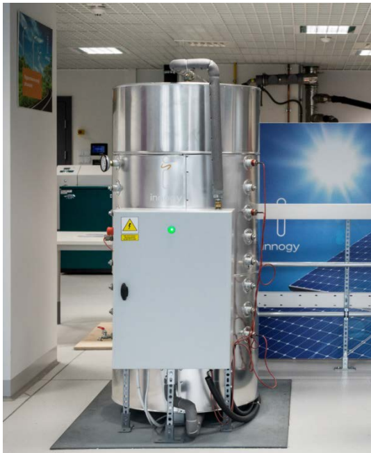
Fig. 7. Thermal energy storage tank.
