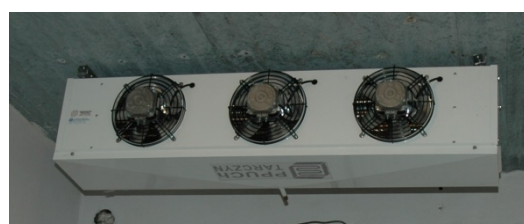
Fig. 1. Front view of the analysed fan-air cooler.
