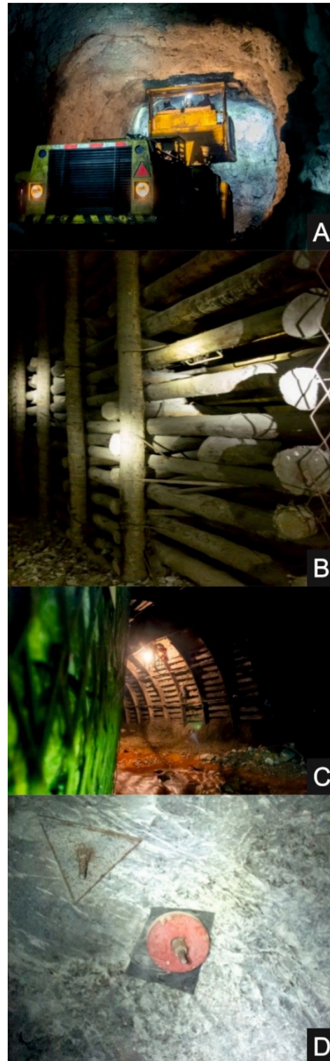
Fig. 2. Additional support of excavations: A) installing of manual rock bolt with steel mesh, B) mining cribs, C) sidewall arch with openwork lagging made by reinforced concrete facing, D) signaling device for roofs stratifications.
