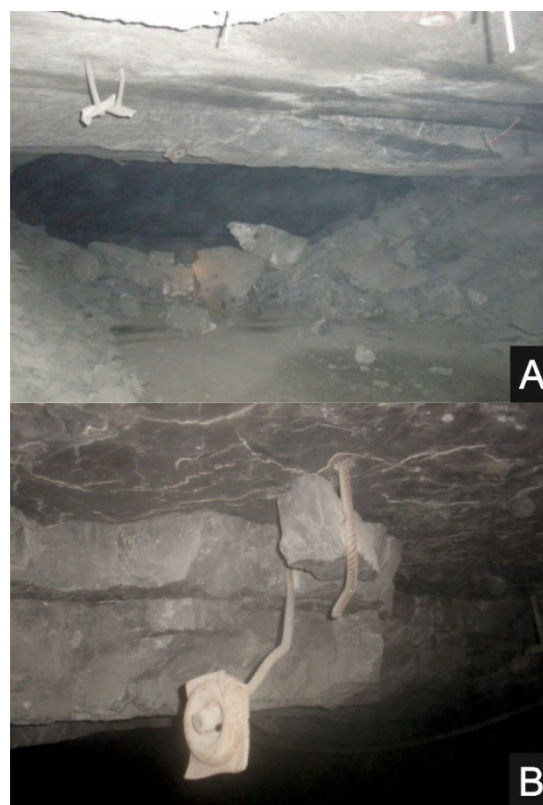
Fig. 1. Roof falls in one of the underground ore mines in the Legnica-Głogów Copper Belt; A) partial filled room by means of roof rocks, B) roof falls of stratificated roof layers.
