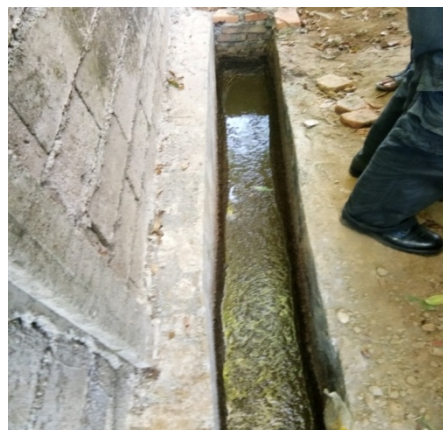
Fig.5. Outlet on Installation
