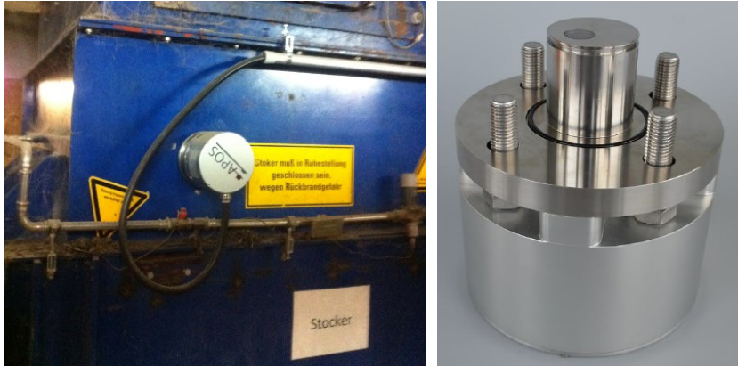
Fig. 9. Measuring head of the Central Spectrometer Unit; installed at biomass hopper at the Scharnhäuser Park (left) and naked (right) [12].
