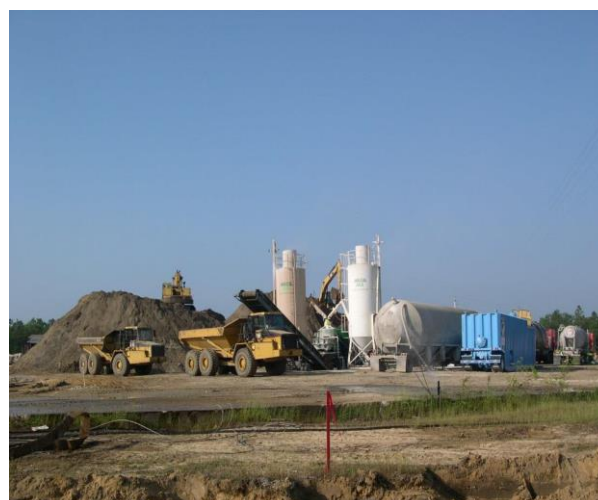
Figure 4. Typical ex-situ S/S equipment, including plant processing, reagent tank, water tank, stacker and haulage
