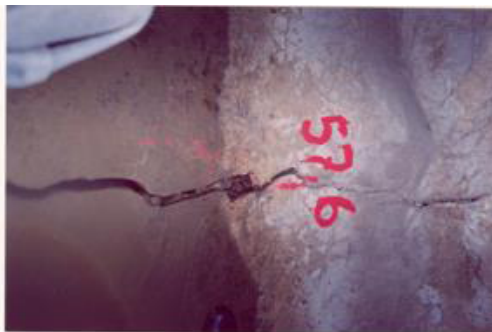
Photo 2. Cracks developed in under ground fish-way.
