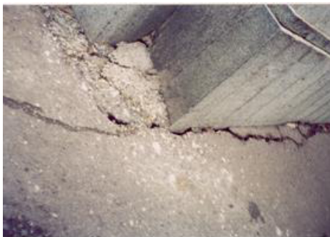
Photo 1. Cracks developed in Ortachala HPP right bank.
