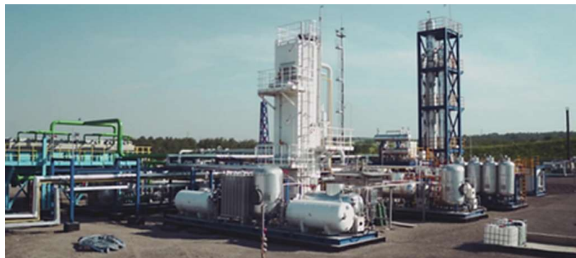
Fig. 1. Natural gas liquefaction plant (Russia, Novokuznetsk, OOO "Siber-Energo").
