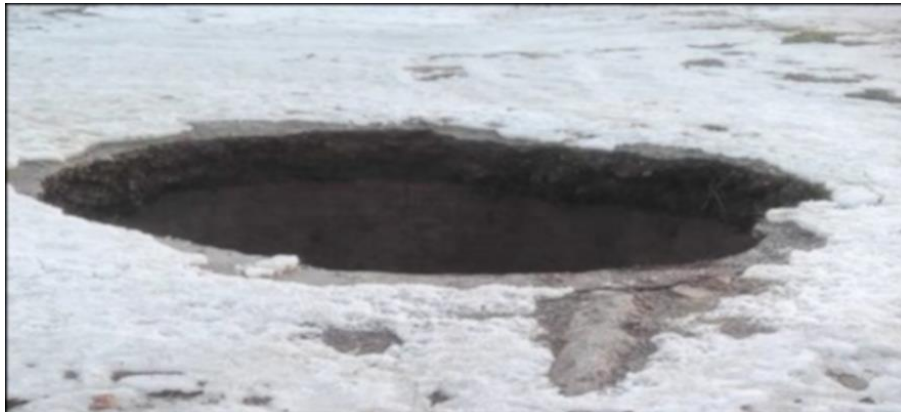
Fig. 2. Open part of the Lubichów III shaft on the day of the mining damage occurrence
