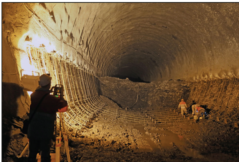
Fig. 1. Works on the installation of temporary lining of the trough part at the stross in the Beskydskyi tunnel (Ukraine).
