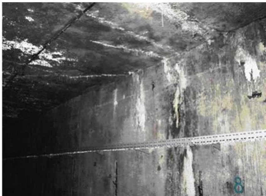
Fig. 1. Cracks with filtration in a concrete timbering of gallery of the Dnistrovskiy hydroelectric power station.
