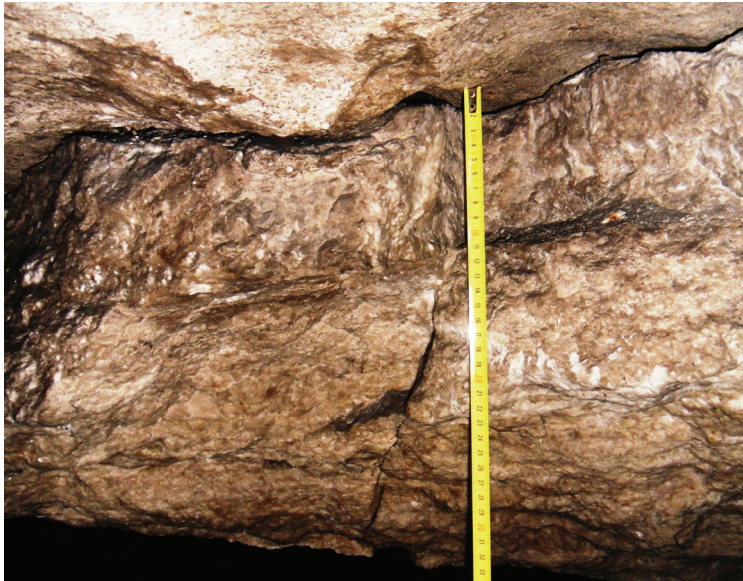
Fig. 3. A photo of separation in a roof of the main transport gallery.
