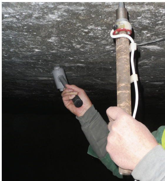
Fig. 4. Realization of vibroacoustic diagnostics of a roof of development by basic option.
