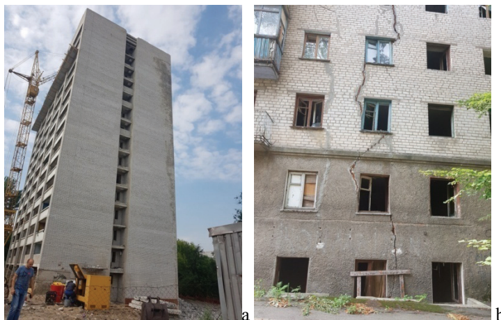
Fig. 7 a, b. Deformations of buildings along the eastern side of the Monastirskiy gully.
