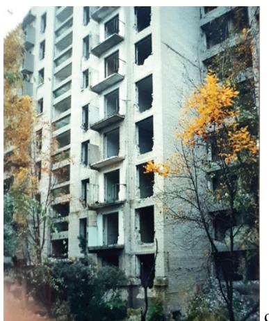
Fig. 7 c. Deformations of buildings along the eastern side of the Monastirskiy gully.
