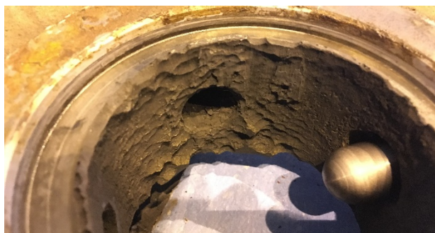
Fig. 1. Photo of corrosion defect of a tool flange.
