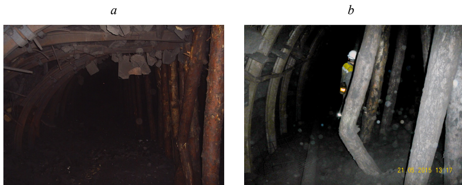
Fig. 3. The fragments of the fastening system state in the preparatory mine working in the zone of the stope works influence during the interaction of the yielding frame of the TSYS type and the rigid (wooden) central prop stay of the strengthening support: a – flattening of the frame cap board and b – destruction of the central prop stays.
