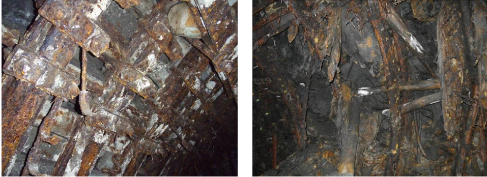
Fig. 1. Corrosion of steel elements (photo M. Rotkegel).
