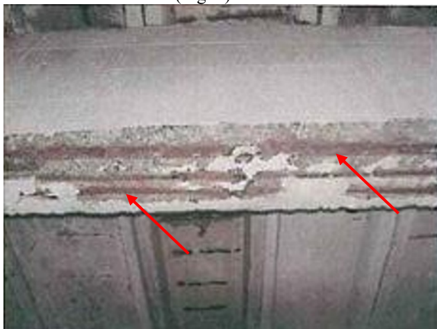
Fig. 1. Corrosion of reinforcement in the beam detected during a technical inspection
