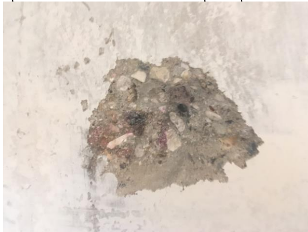
Fig. 2. The absence of visible signs of concrete carbonation according to the phenolphthalein test
