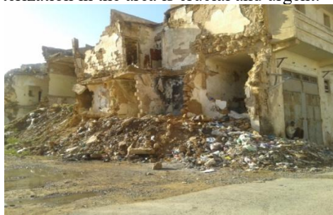
Fig. 1. Degradations observed in the coastal part of Safi.
