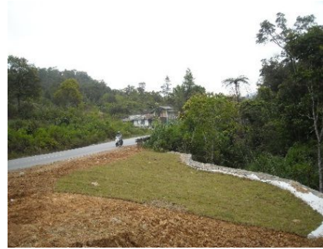
Fig.7b. The gabion retaining wall after sliding
