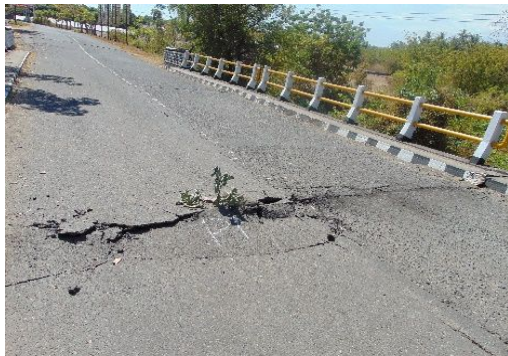
Fig. 2. Damage at the expansion joint in LUK bridge [7]
