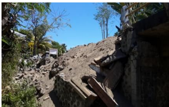
Fig. 1. Subsidence of embankment near the Tampes bridge [7]
