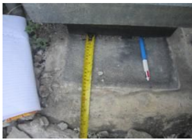
Fig. 3. Excessive superstructure displacement in Batusuya bridges [8]
