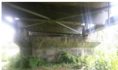
Fig. 4. Settlement of pier foundation in Tompe bridge [8]
