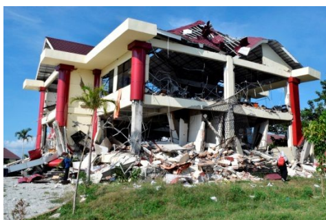
Fig. 4. The Dean Building of the Faculty of Social and Political Science (FISIP) of Tadulako University in Post-Earthquake 2018
