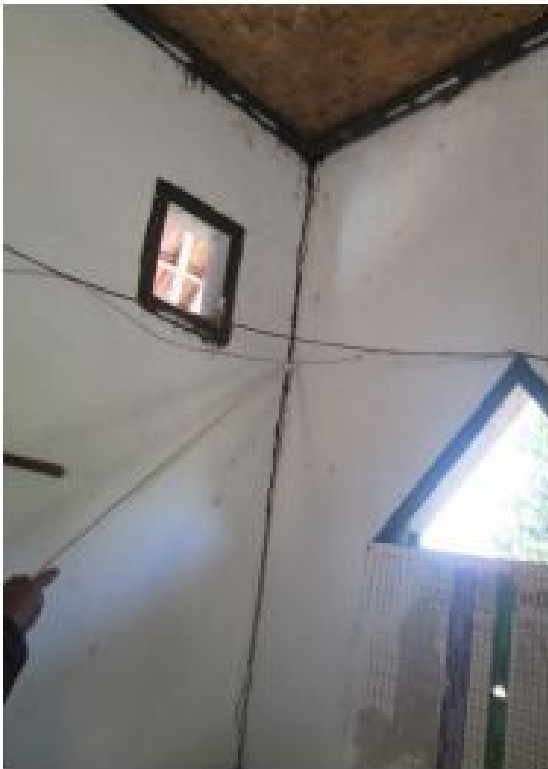
Fig. 6. The Damage type of SD 02 Obel-obel
