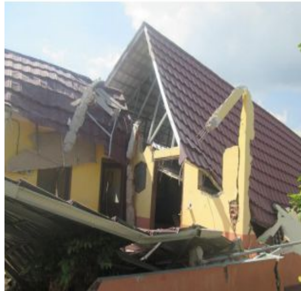
Fig. 8. The total damage structure of Paud Terpadu PB
