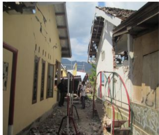
Fig. 9. The Heavy Damage type of Paud Terpadu PB
